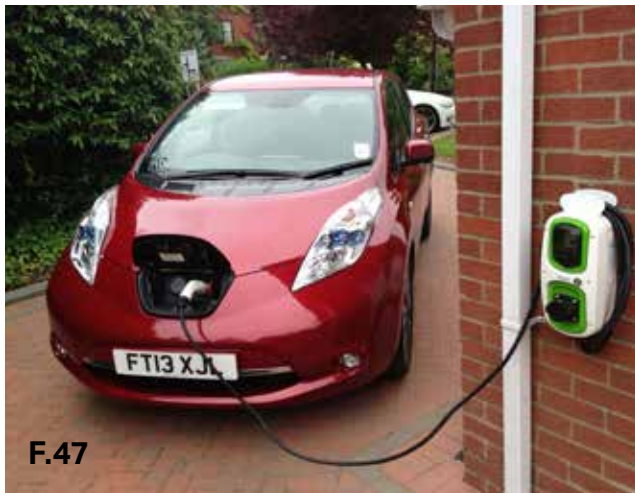
Figure 47: Off-street mounted car charging point
