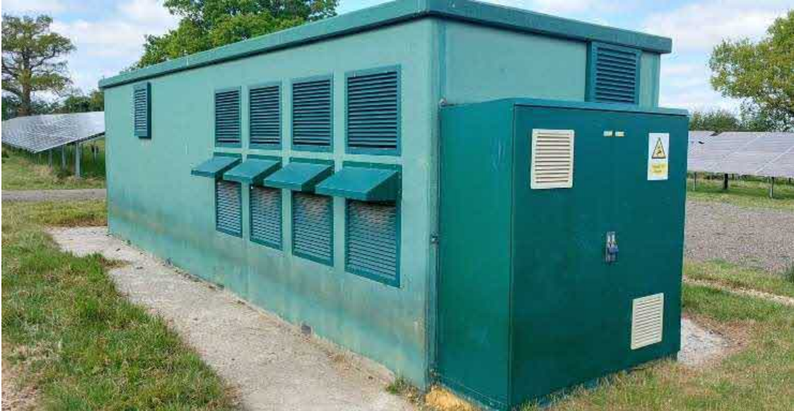
Plate 3: Typical Inverter Station facility
