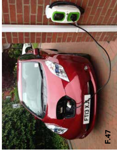
Figure 47: Off-street mounted car charging point
